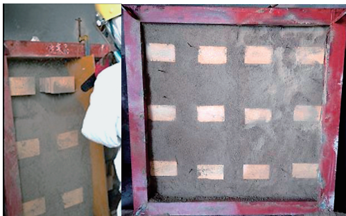
Fig. 7 Appearance of large-sized panel with anchor bricks used for simulative gunning experiment.
